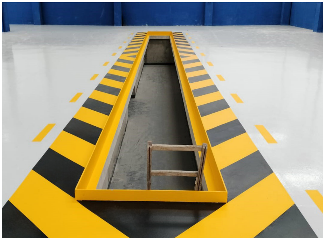
EP 10 SYSTEM: MECHANICAL WORKSHOP. SPAIN
